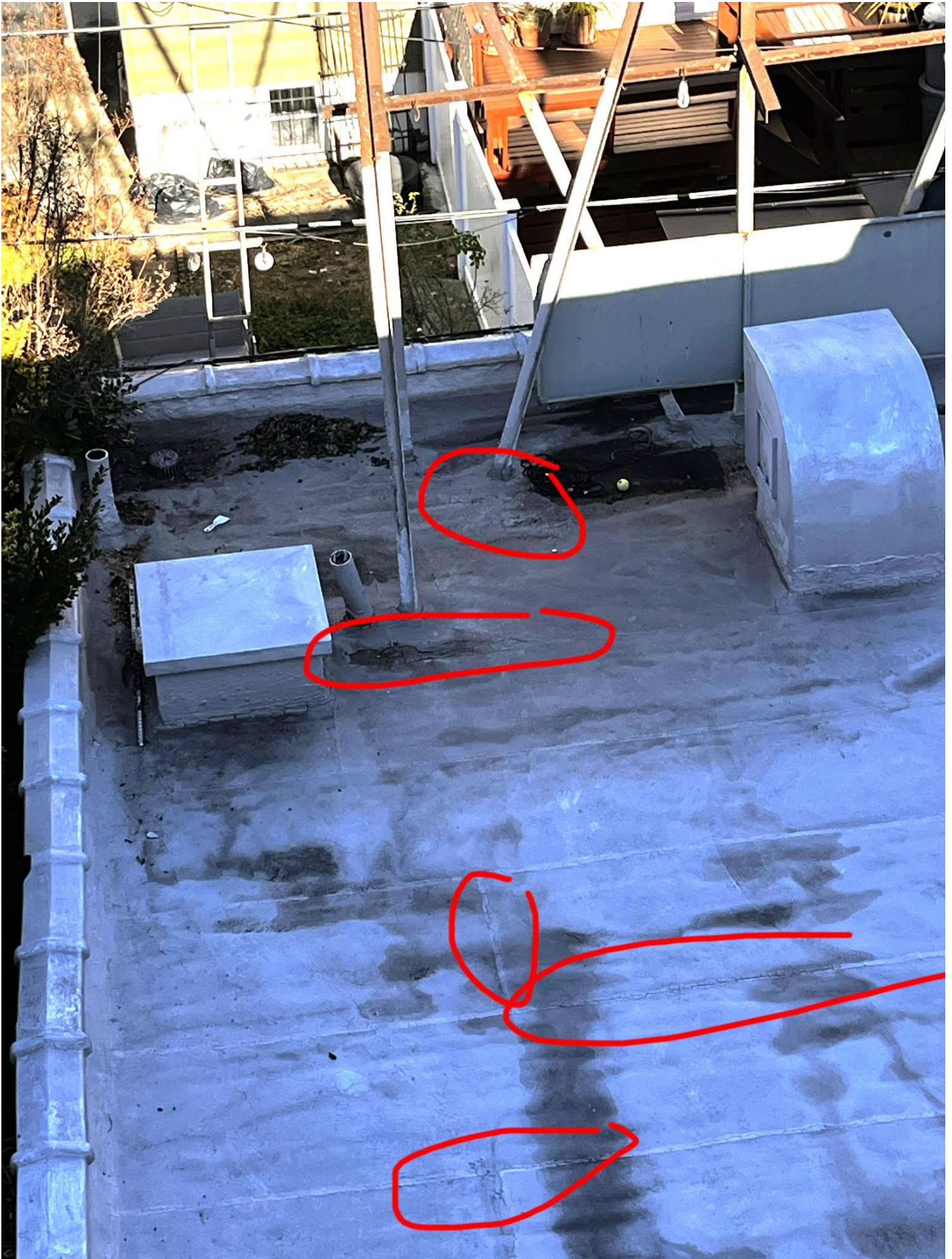
Visible cracking on much of roof, even from far away.
