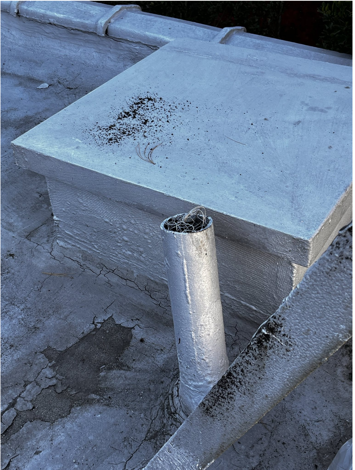
Cracking, cleaning, and vent pipes need covers.
