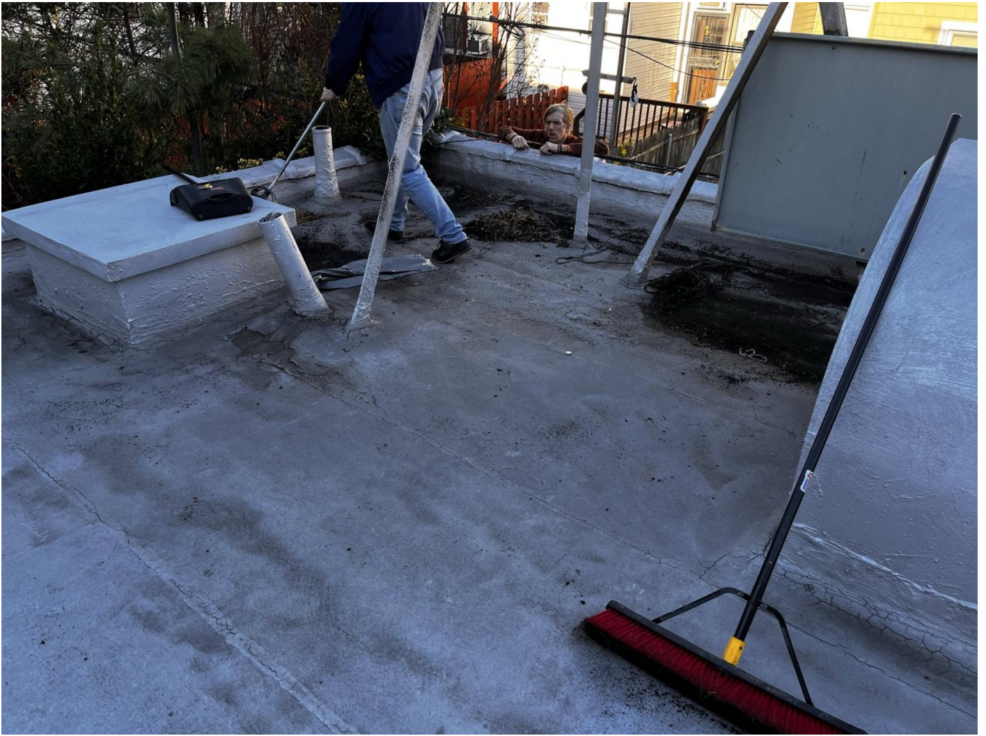
Some areas would benefit from regular leaf/debris cleaning
