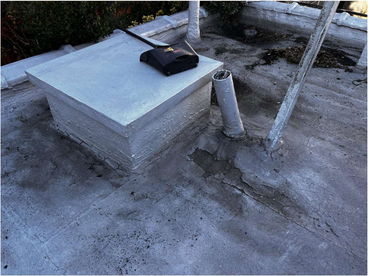
Cracking, cleaning, and vent pipes need covers.
