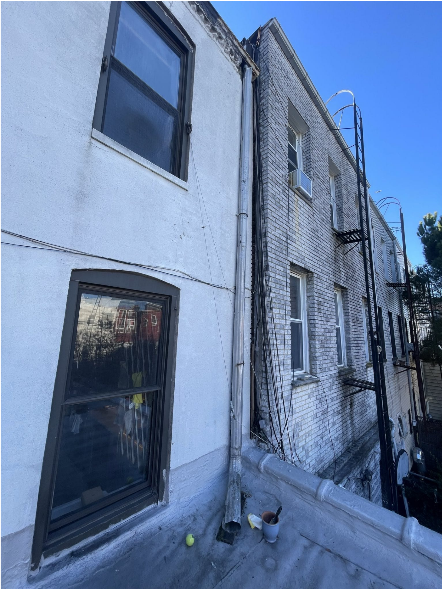
Top roof downspout drains to lower roof, possible to direct to drain outside building?
