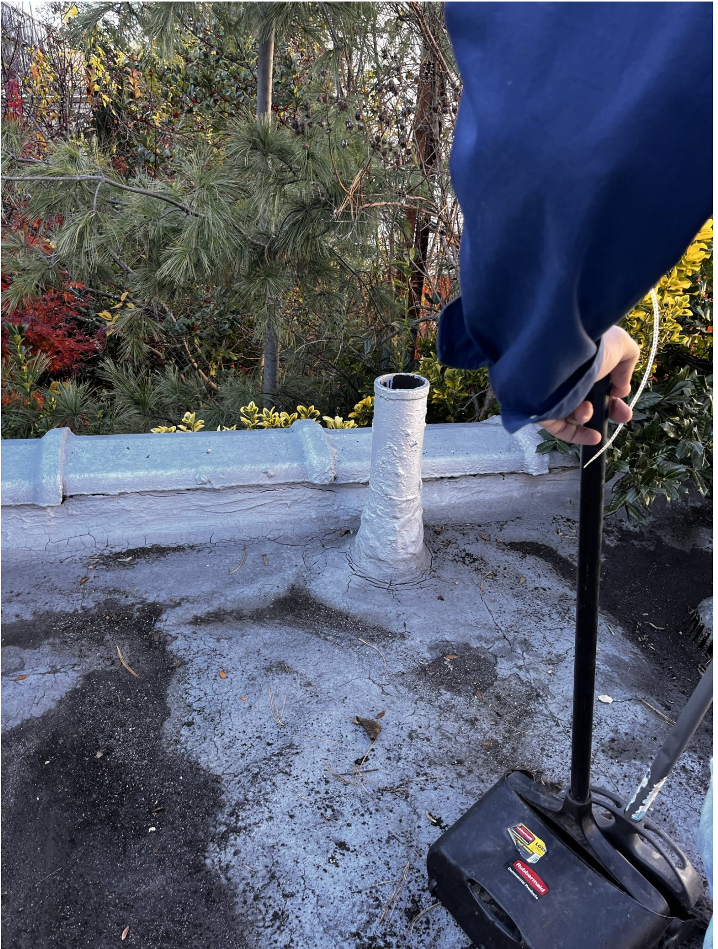
Cracking, cleaning, and vent pipes need covers.
